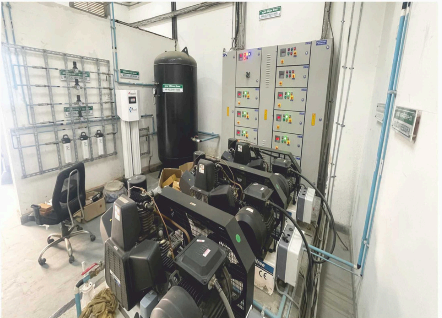
Medical Air Plant
